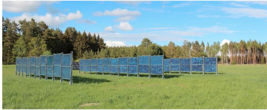
Figure 2.4 Vertical bifacial agrivoltaic system in Sweden (Campana, 2021)
