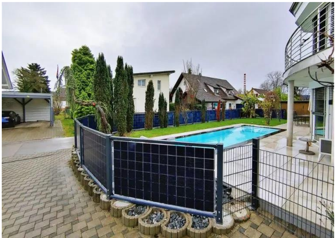
Figure 2.5 Solar Fence manufactured and installed by Next2Sun (Next2Sun, 2024)
